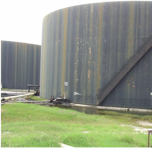
View of existing HFO Storage Tank No. 112
