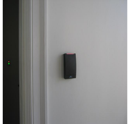
Access Control Unit installed inside the Port Authority of Jamaica Head Quarters at Falmouth Cruise Ship Pier
