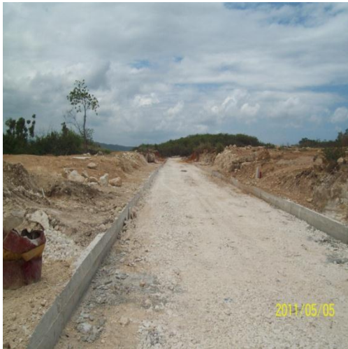
Incomplete Infrastructure Works
