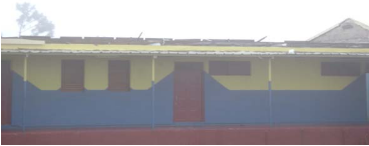
Manning's Boys Home in December 2007 after Hurricane Dean
